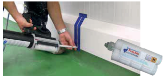
POLYSTO OP30RB SANICOAT WITH EPOXY FLOOR COVING APPLIED INTO A REBATE AND FINISHED WITH POLYSTO HYGISEAL.
